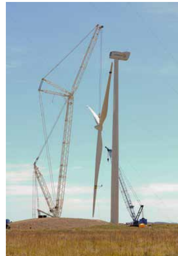
Towers are being lifted as work continues on the 2 MW Gamesa wind turbine that is being installed at the NWTC. Credit: NREL
